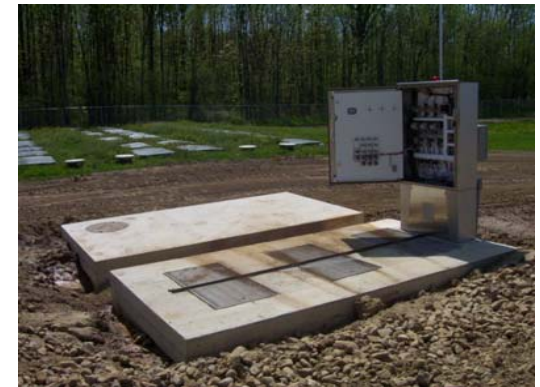
Shenandoah Area Pura-flo Wastewater Treatment System, Richland County, Ohio
